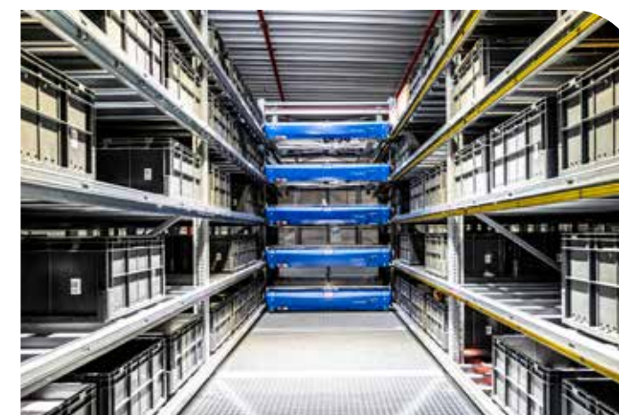
Roughly 170 Stingray systems are currently in operation in the nine-aisle shuttle warehouse.
